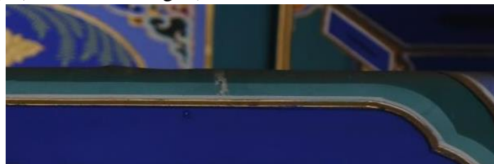
Fig. 4 Eaves - animal damage
