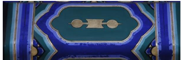
Fig. 2(2) Outer Eaves - Loss of paint
