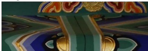
Fig. 3 (1) Inner Eaves - Dust accumulation
