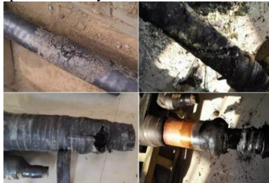
Figure 1: Cable insulation breakdown photos
