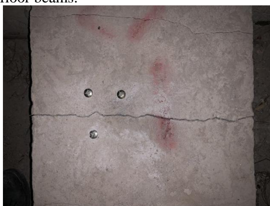
Figure 2: Tension Failure of Connecting Beams
