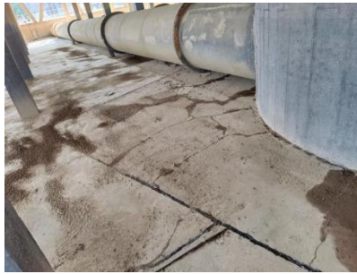
Figure 4: Indoor Floor (Pool Bottom Plate) Crack
