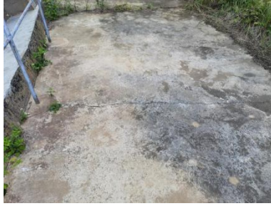
Figure 3: Outdoor Floor Crack 2
