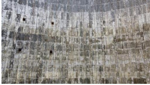
Figure 6: Scale on the Inner Wall Concrete Surface of the Shell
